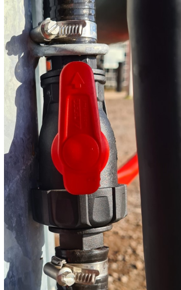
Filter Valve open, flow from pump going to chemical mixer.
