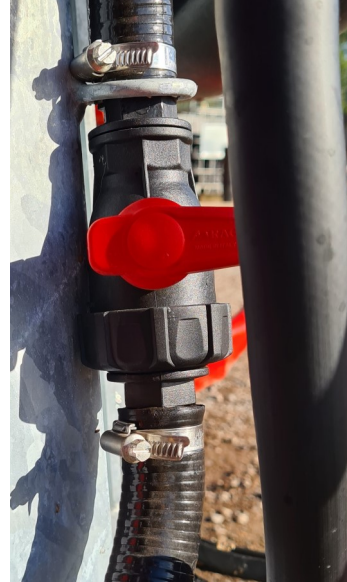
Filter Valve closed, chemical mixer isolated. Valve should be in this position when three way valve is in A. WORK mode.
